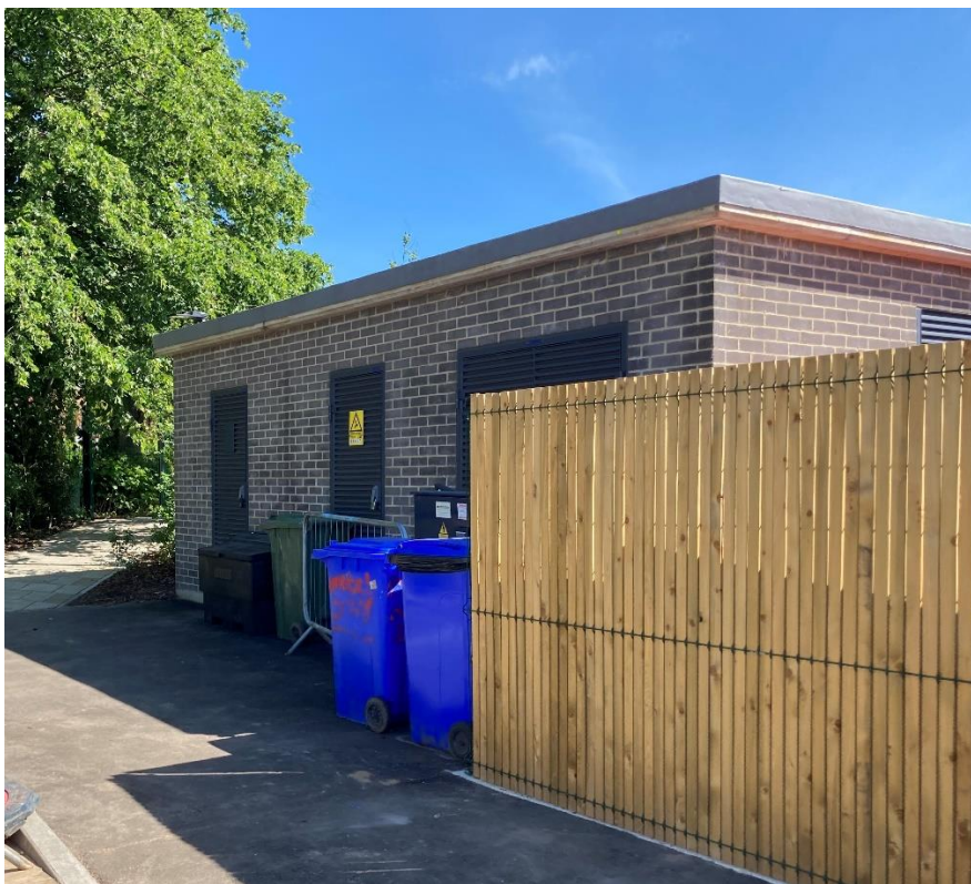
Fig 3: Sub-station, as built, viewed from within the site
